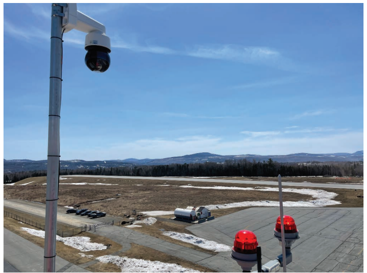
A LifeFlight weather camera was installed overlooking the runway at Stephen A. Bean Municipal Airport in Rangeley in March 2023.
